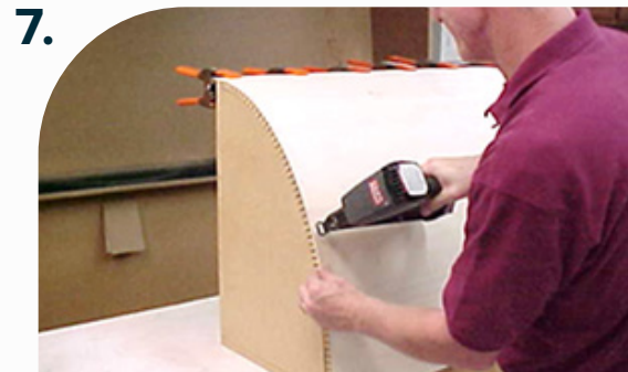
Staples can be used on the outside face along ribbing. Face is now ready for lamination.
